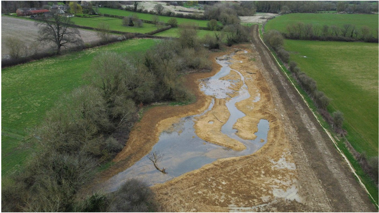
Cornwell Estate River Restoration: Top section involving excavation of channels and exposing subsoil and gravels. Drone footage [Wild Oxfordshire]
